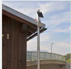
Sensor installation in gauge station or in observation wells in the water. RTU with solar panel attached to a mast.
